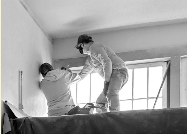
Roger Betschler and Michael Bednarski insulate the windows above our show windows.
